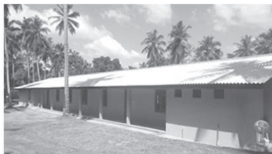
The building which is being under construction donated by Ven. Pannila Sri Ananda Thero...
